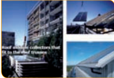
Solar collectors avoiding to repair a terrace roof
